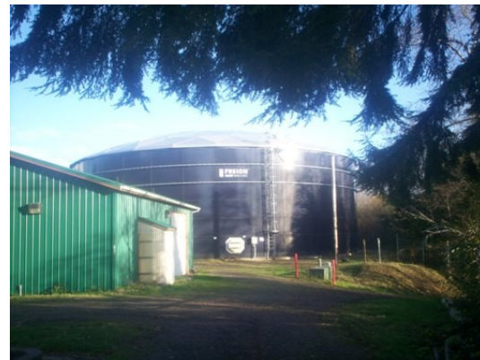
City of Nehalem Water Treatment Plant & Reservoir
